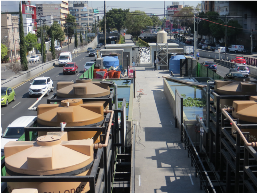
← Tanks to process sewage and remove toxic material.
