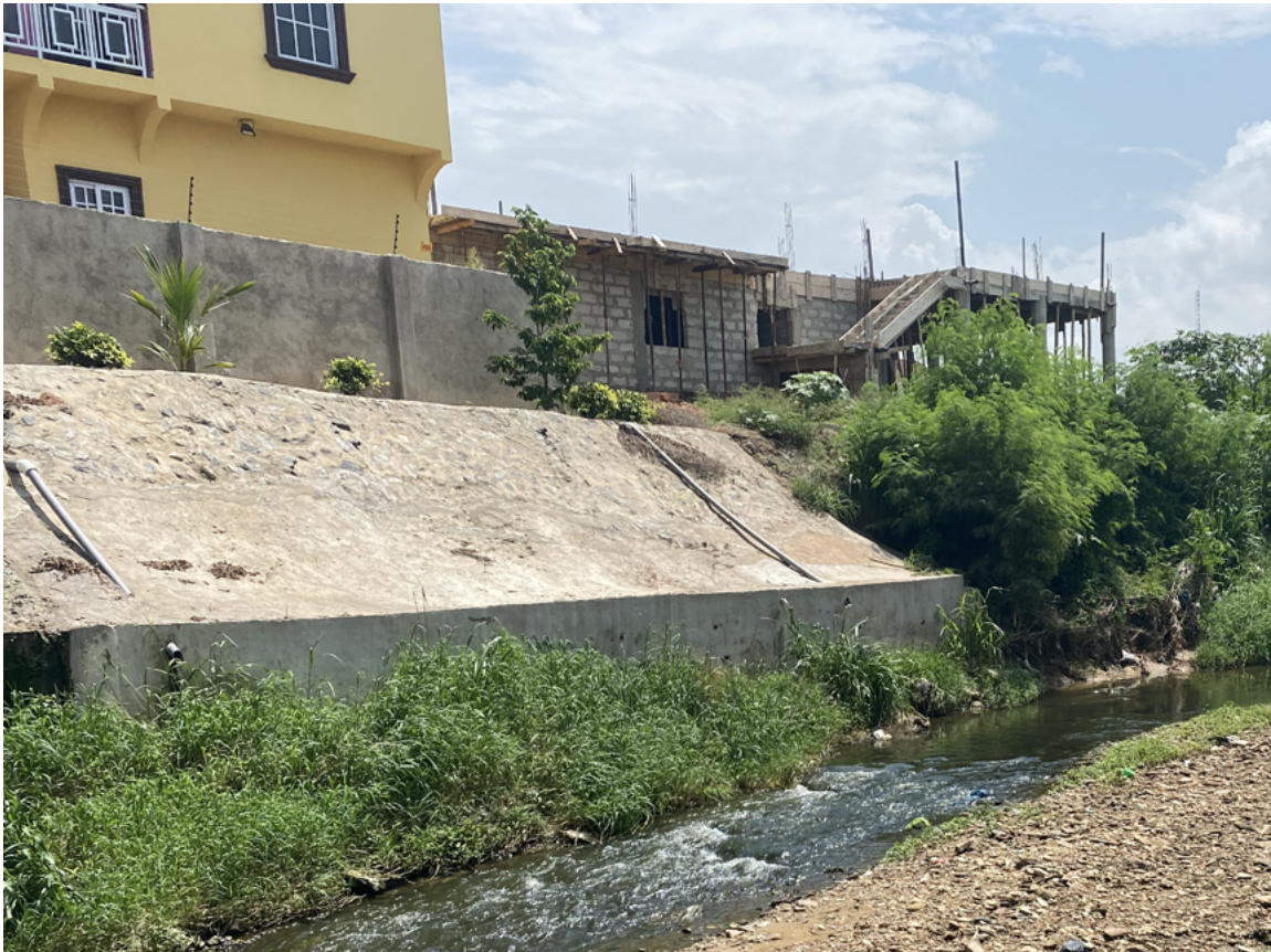
Flood barrier in the mid-stream and mixed-income East Airport neighborhood, Accra. Photo: Afra Foli, 2020.
